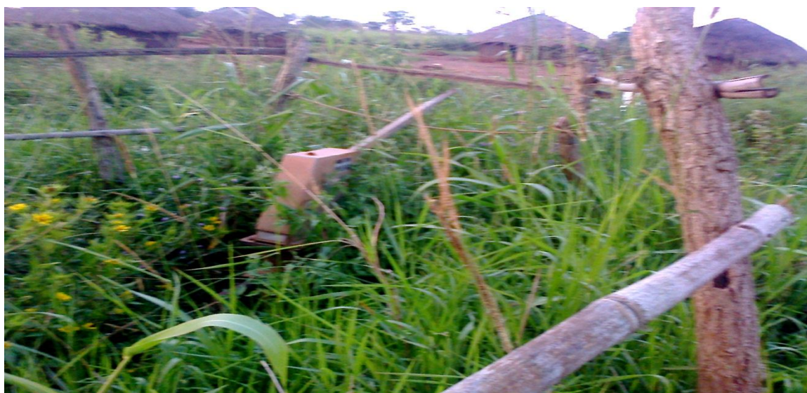
Figure 3: Non- functioning borehole in Abili village
